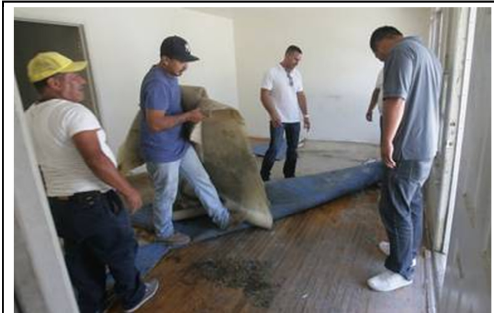
Jimmy Previti, middle, with Frontier Enterprises, stands in a bank-owned home he acquired to fix up and re-sell. From left to right are workers Francisco Perez, of Chino, Edwin Garcia, of Fontana, Previti, and construction manager John Chon.
