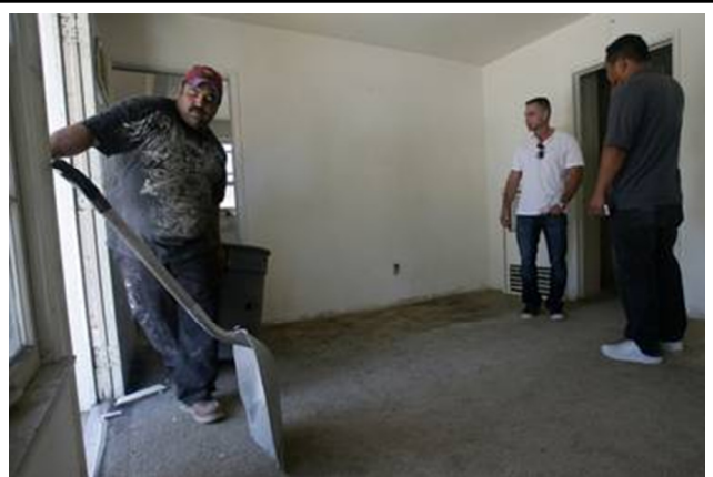
Jimmy Previti, middle, with Frontier Enterprises, stands in a bank owned home he acquired to fix up and re-sell Friday. With him is Jose Garcia, of Riverside, left, as he removed debris from the home and construction manager John Chon, right.
